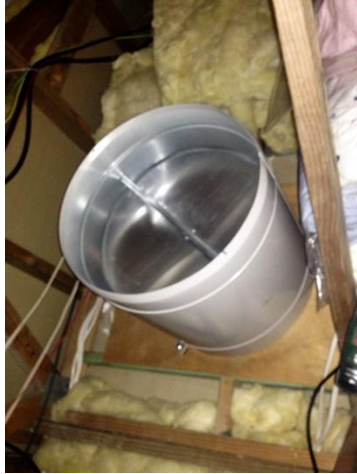
Figure 5. Damper in position.
