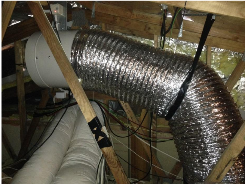
Figure 1. Installed prototype at my house in Chapel Hill.
